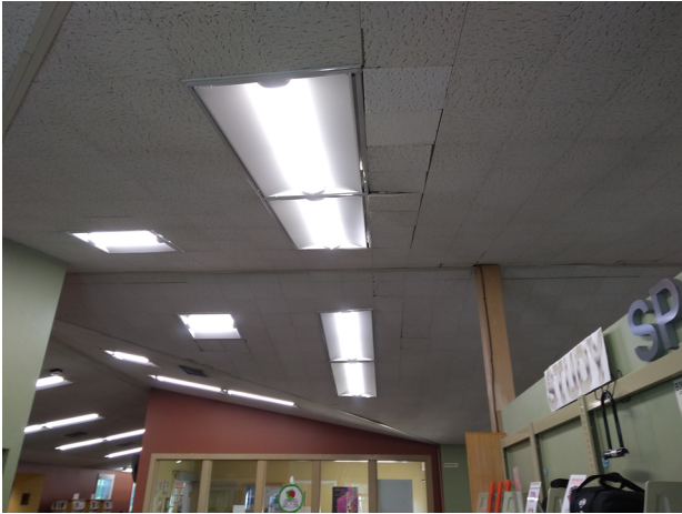
1. Splined acoustic ceiling tiles are stained and delaminating.
