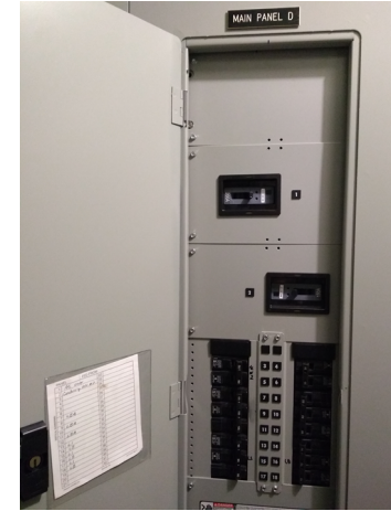
3. Multiple electrical panels in several locations.
