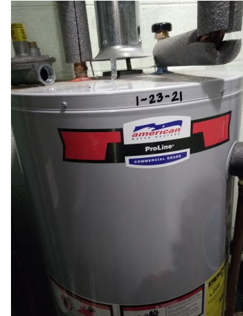
6. Gas water heater was replaced in 2021. Assume 10-year life expectancy.
