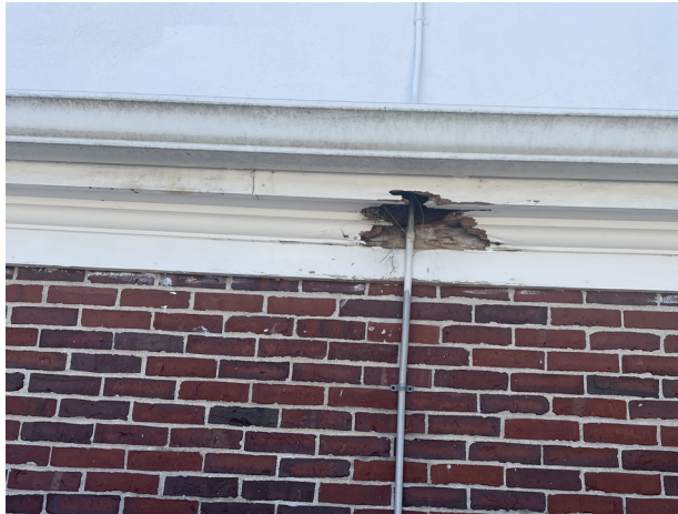
11. Animals have gained access to eaves.
