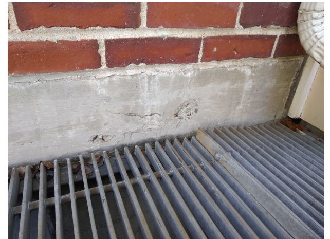
6. Concrete is spalling and re-bar is exposed on foundation walls in several locations.
