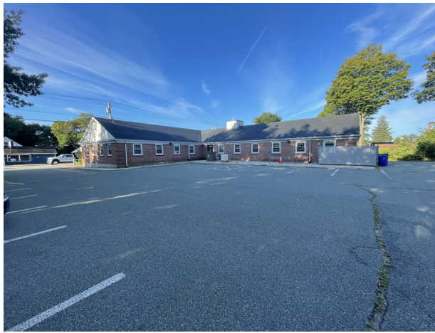
2. Bituminous at parking lot has deep cracks.
