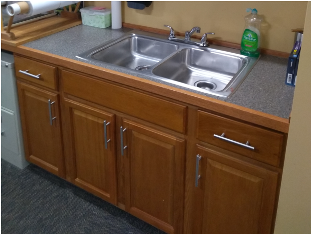
4. Sink in Work Room is not accessible.
