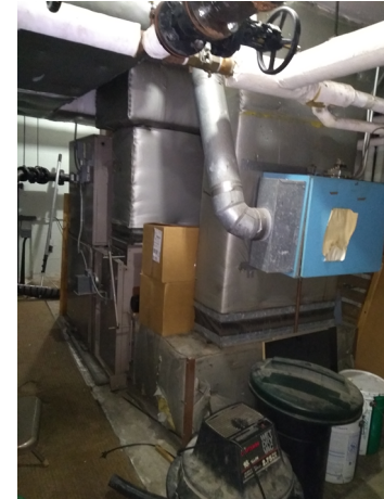
3. Existing ventilation and HVAC system is inoperative.
