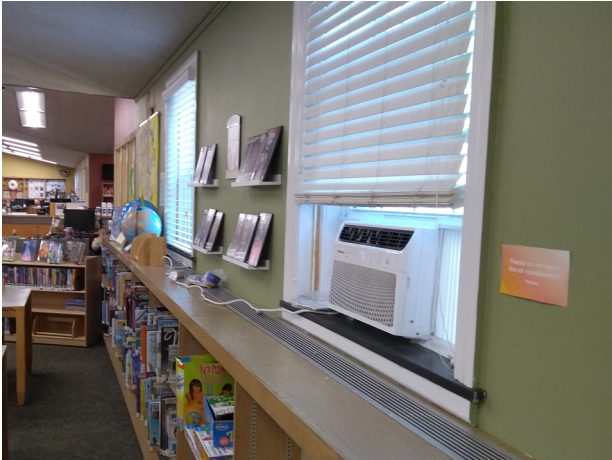
1. Window air conditioning units are not providing adequate cooling.
