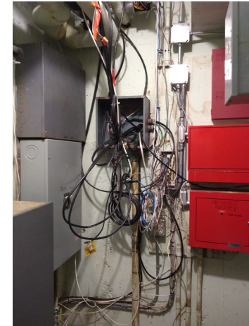
6. Various information technology systems have been abandoned in place.
