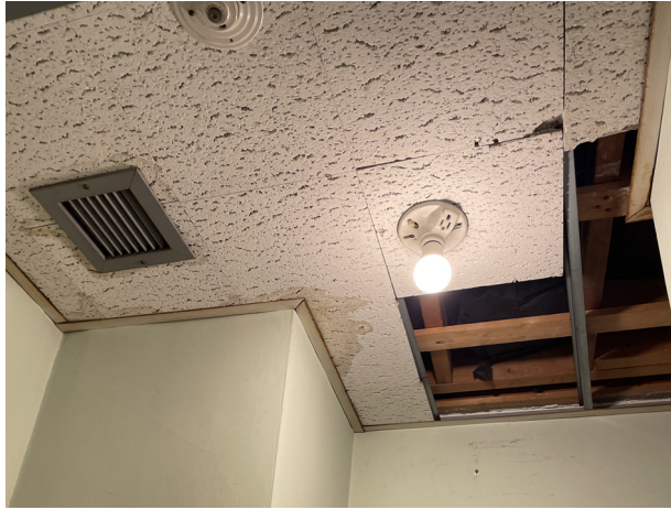
2. Splined acoustic ceiling tiles are damaged, stained, and outdated lighting is inefficient.
