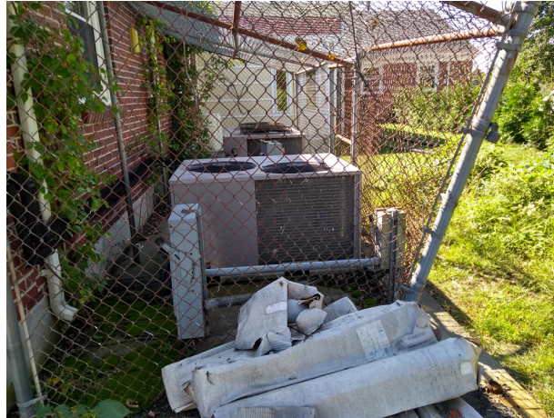
2. Existing ventilation and HVAC system is inoperative.
