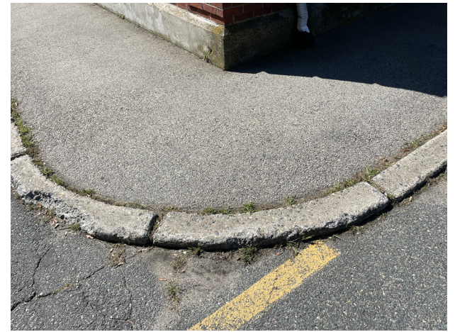
3. Concrete curbs are damaged.
