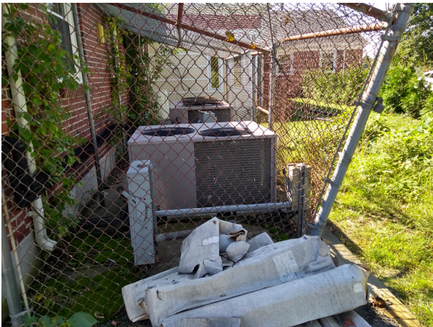
4. Chain-link fence enclosing mechanical equipment is damaged.
