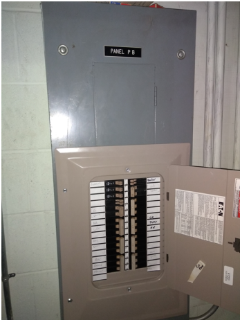
4. Multiple electrical panels in several locations.
