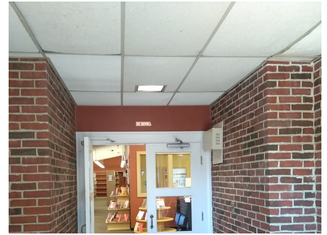
3. 2' x 4' acoustic ceiling tiles are warped and sagging.
