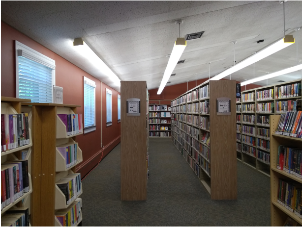
1. Fluorescent light fixtures are inefficient.
