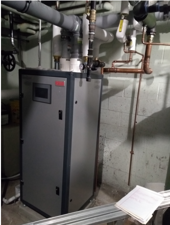
4. Gas boiler replaced in 2021. Assume 20-year maximum life expectancy.
