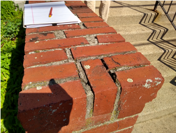
10. Mortar is damaged at brick wall at south stairs.
