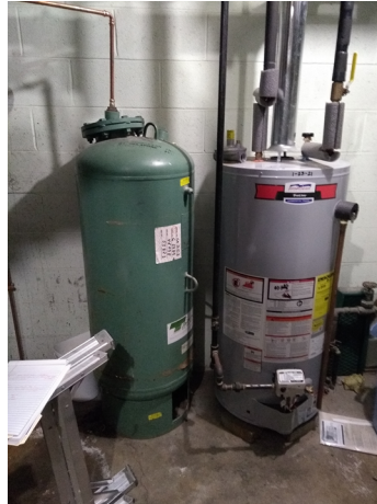
5. Expansion tank is an older unit but appears in good condition.
