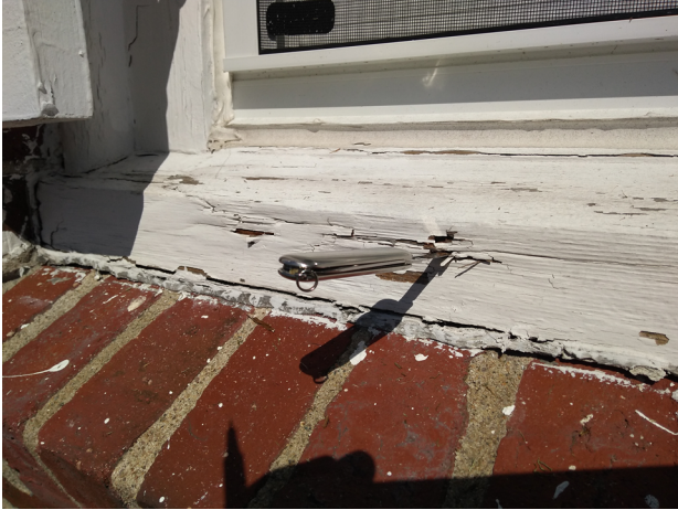
7. Wooden windowsills are decaying.
