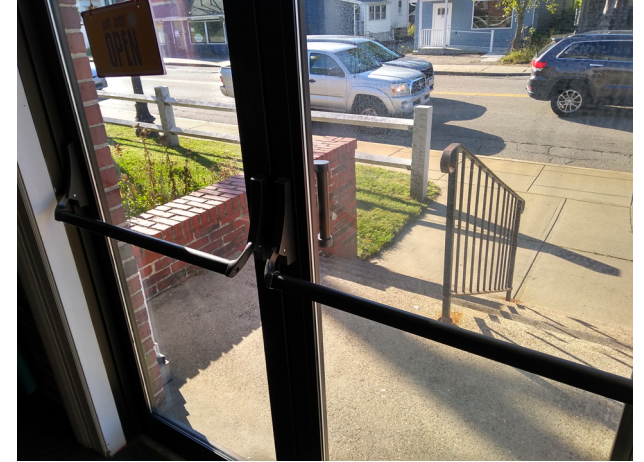
9. Exit doors at 30" wide and metal handrail do not meet MAAB requirements.
