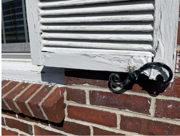
8. Wood shutters are decaying.
