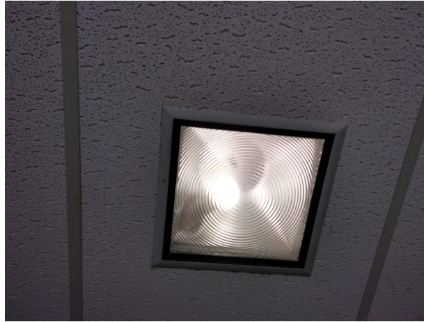
2. Outdated light fixture.
