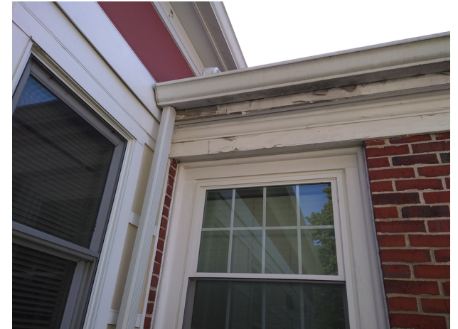
12. Paint is peeling at wood surfaces.
